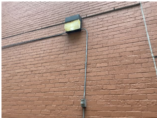
Lighting Fixtures - Exterior - HID Wall Packs
