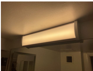
Emergency Battery Lamp Ballast
