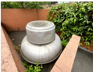
Exhaust System - General Building and Restroom
