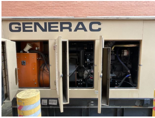
Emergency Generator - 150 kW
