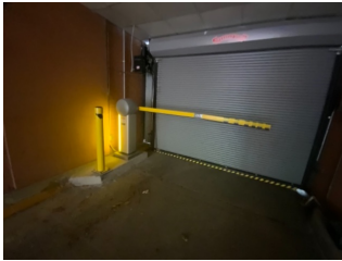
Parking Equipment - Ticket Spitter and Gates Parking Equipment
