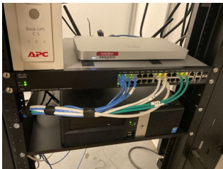
Security System - CCTV Video - Average Density - New
