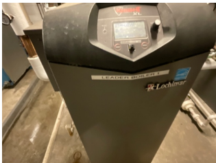
Water Heater - Gas - Comm - 700 MBH (x2)*
