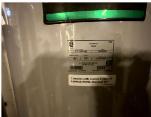
Domestic Water Storage Tank - Galvanized Steel - 120 Gal (2X)
