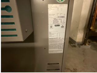
Water Heater - Gas - Comm - 700 MBH (x2)*
