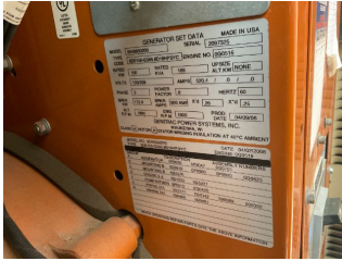
Emergency Generator - 150 kW
