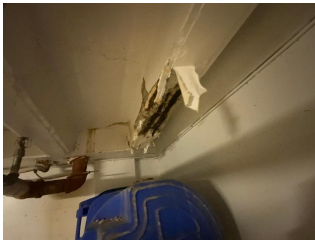
Exposed and Rusted Reinforcement
