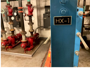
Heat Exchanger - Condenser Water
