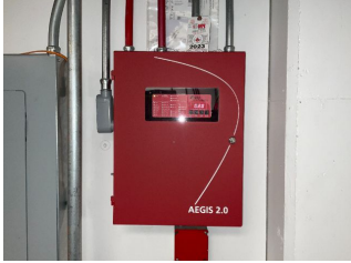
Fire Alarm System - FACP
