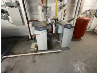
Water Heater - Gas - Comm - 700 MBH (x2)*
