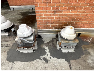
Exhaust System - General Building and Restroom
