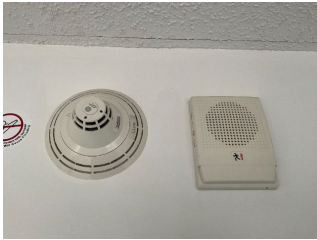
Fire Alarm System - Initiating & Alarm Devices
