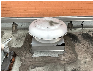
Exhaust System - General Building and Restroom
