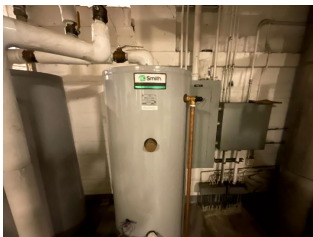
Domestic Water Storage Tank - Galvanized Steel - 120 Gal (2X)
