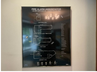
Fire Alarm System - Initiating & Alarm Devices
