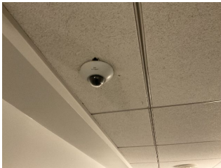
Security System - CCTV Video - Average Density - New
