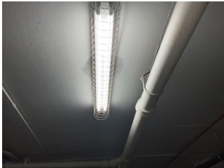
Lighting Fixtures - Interior
