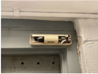
Security System - Access Control System
