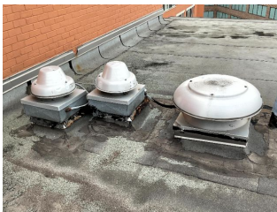
Exhaust System - General Building and Restroom
