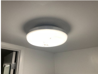
Lighting Fixtures - Interior
