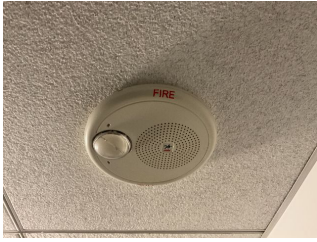
Fire Alarm System - Initiating & Alarm Devices
